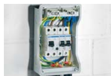
British Standard installation with earthed armored cables
